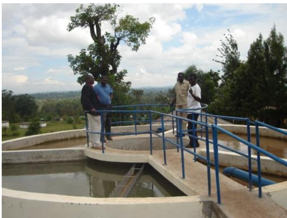
Figure 6: A new clarifier constructed with funding from the SMM project at Angurai Water Treatment Plant in Western Kenya.
