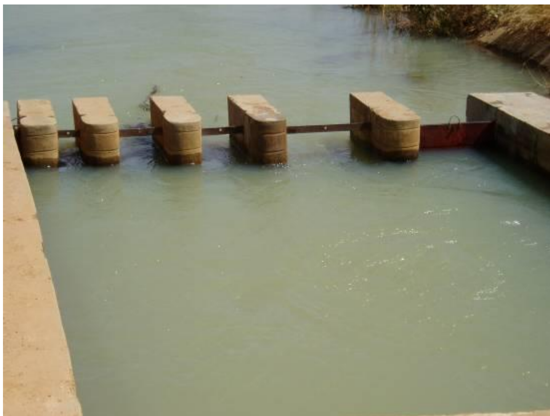
Plate 5: Kadawa Sector Turnout with missing metal shutters
